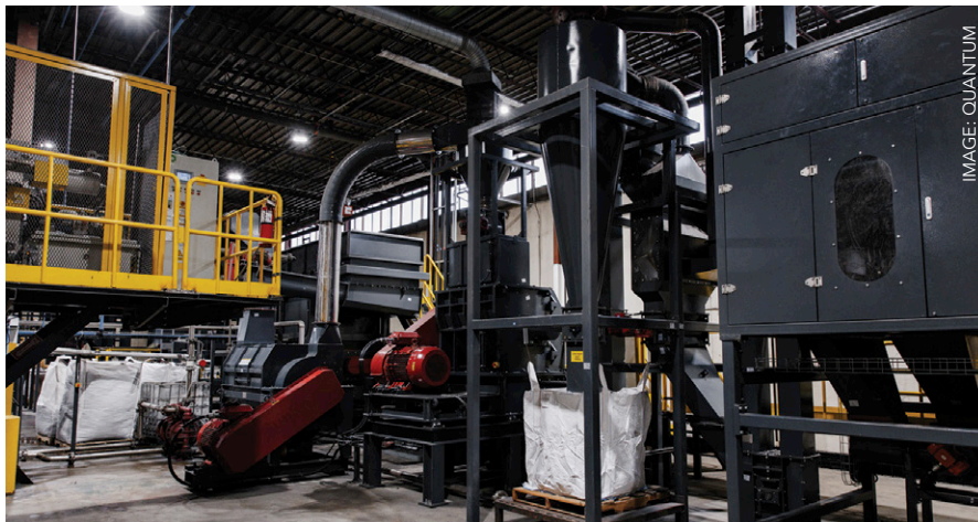
Quantum Lifecycle Partners installed the line at its facility in Toronto, Canada
